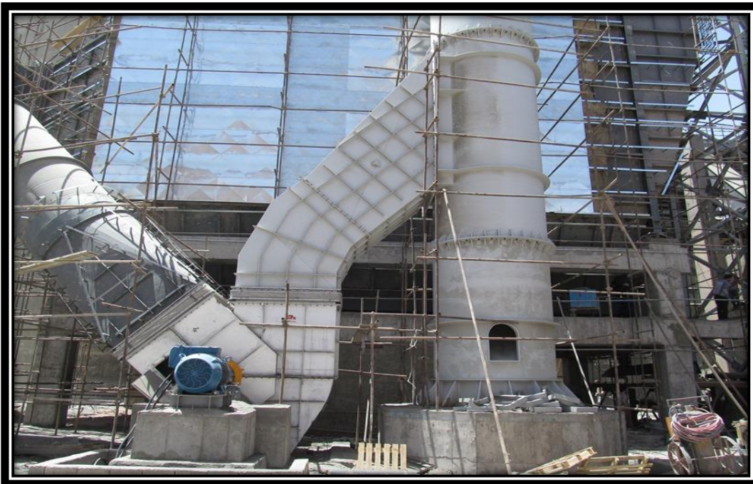
Electrofilter project of Kerman Cement Company
