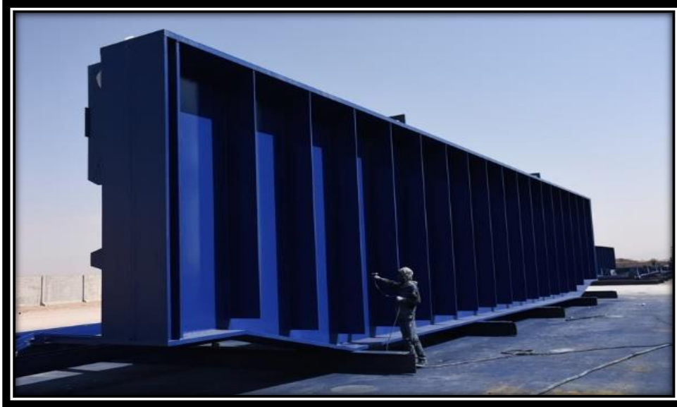
Construction and painting of a 28-meter crane beam by Shokofa Sanat Poya Company
