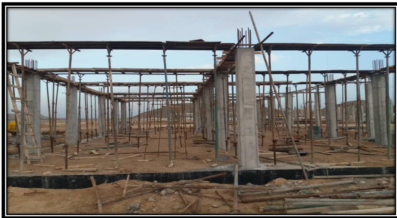
Implementation of piling and preparation of workshop conditions for the reinforcement of roof elements (Ferrosilicon factory construction project)
